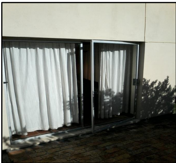
Figure 12: Sliding door pulled off rails by GOB5
